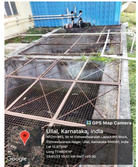
Treated water tank
